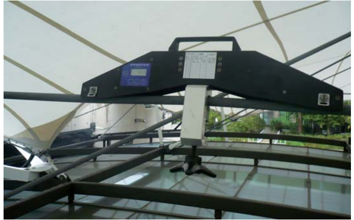
Determination of the cable forces using a measuring gauge for cable tension from PFEIFER Seil- und Hebeteknik GmbH
